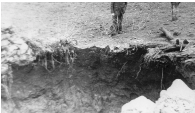
Fig. 4 Surface subsidence above ventilation adit
