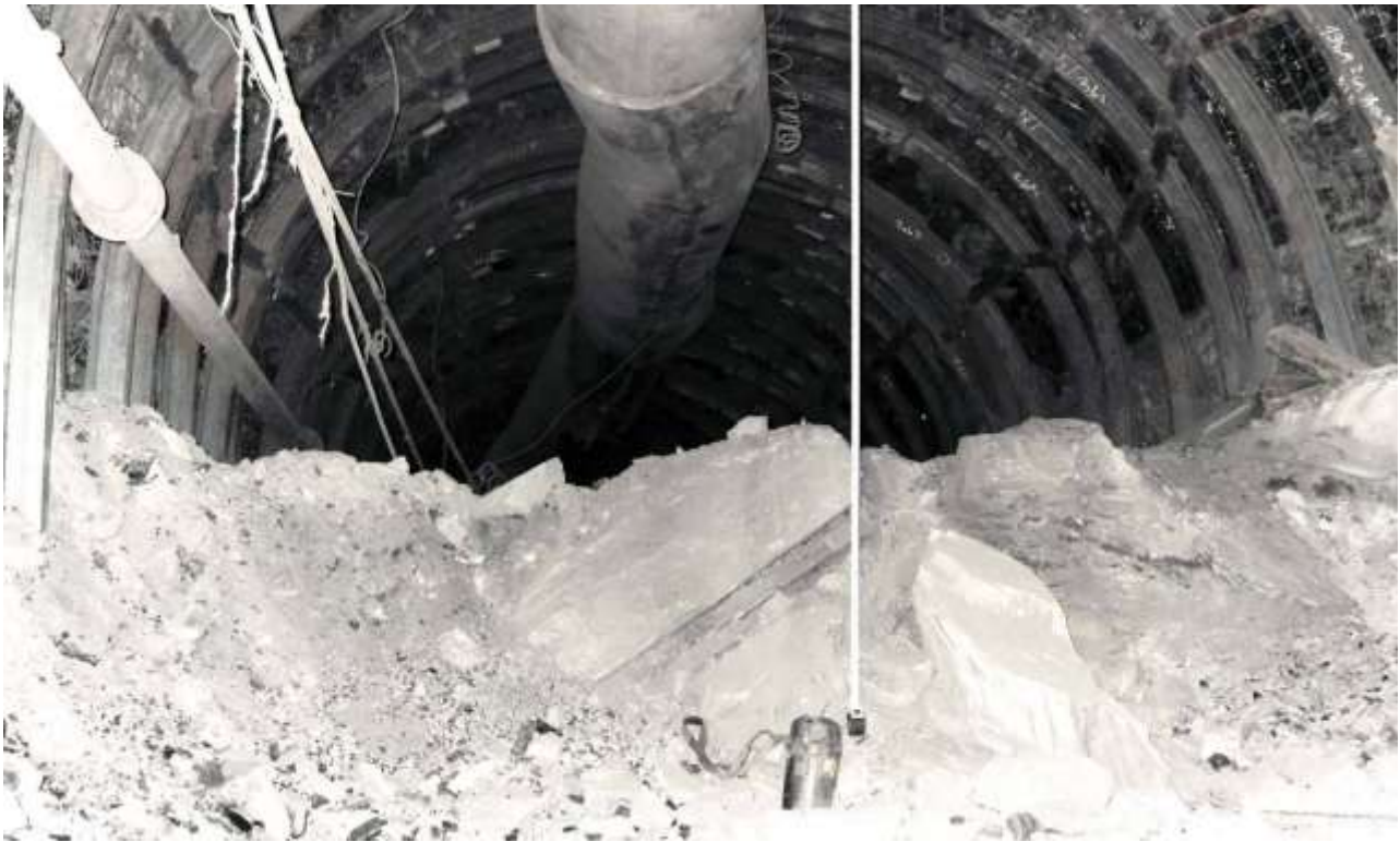
Figure 1 – Nature of look of a rock floor heaving in 8 th east belt entry seam m_3
